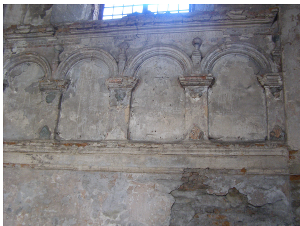
Fig. 6. Synagogue in Zhovkva. Fragment of blind-arcade belt under the windows of the prayer hall: photo taken in 2008.
