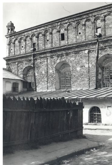
Fig. 8. Southern wall of the synagogue, with traces of demolished span roofs of the synagogue annex: from the collection by S. Kravtsov (Jerusalem).
