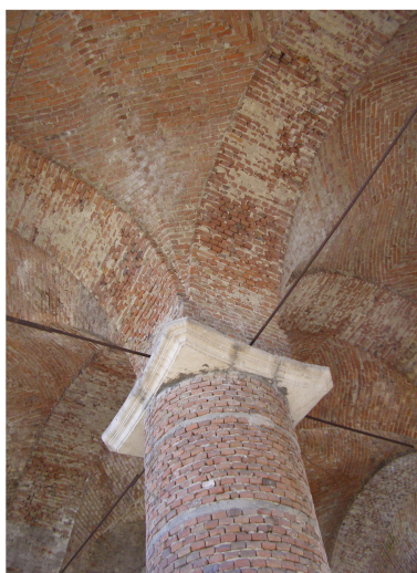
Fig. 33. A column and an arch of the main prayer hall reconstructed in 1955–1956: photo taken in 2008.
