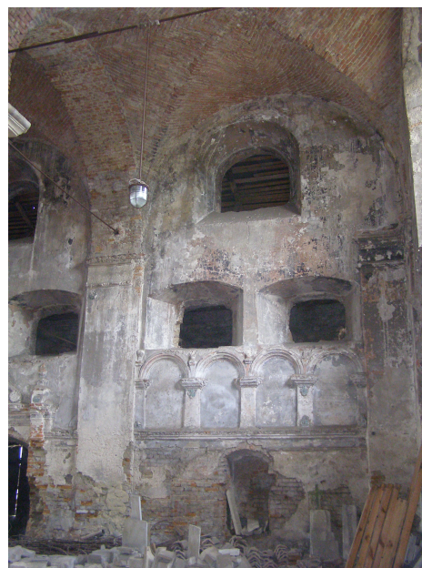
Fig. 10. View of the western wall. Blind-arcade belt cut by chopped holes of the women's gallery: photo taken in 2008.
