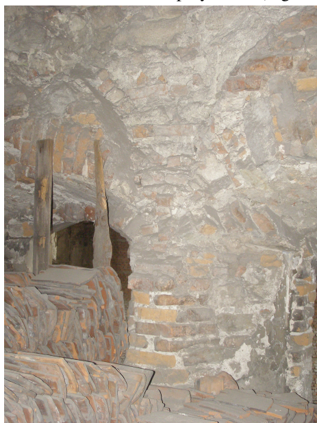
Fig. 9. Traces of rebuilding of wall of the western synagogue's body: photo taken in 2008.
