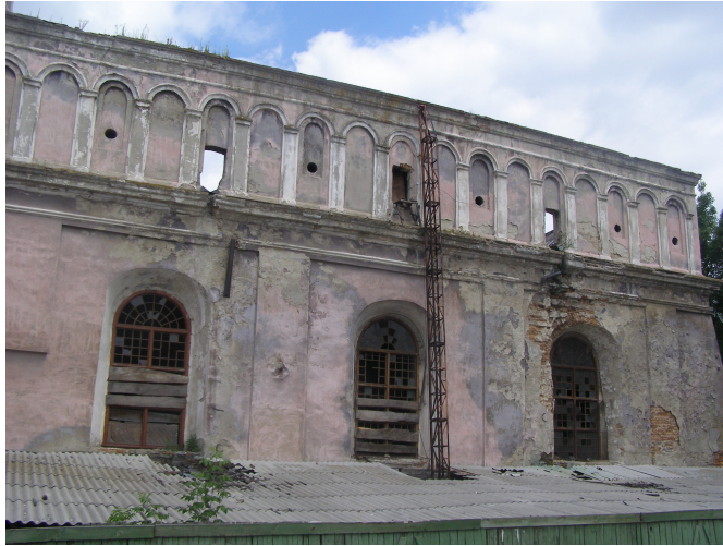
Fig. 18. Synagogue in Zhovkva. Southern facade. Openings in the windows reveal signs of lowering: photo taken in 2008.
