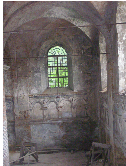
Fig. 20. Fragment of interior of the synagogue that includes an extreme window, of which axis does not coincide with the axis of the vault: photo taken in 2008.
