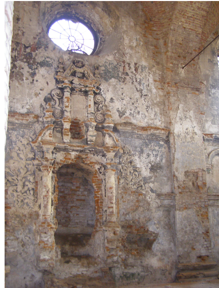
Fig. 36. Synagogue in Zhovkva. A preserved niche of Aron Kodesh at the axis of the eastern wall of the prayer hall: photo taken in 2008.
