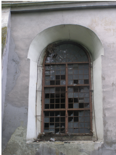
Fig. 19. Traces of lowering of a window on the northern facade: photo taken in 2008.
